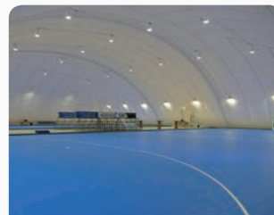
RSI installed total-concept at HOD Valkenswaard, which includes flooring and LED floodlights as well.
